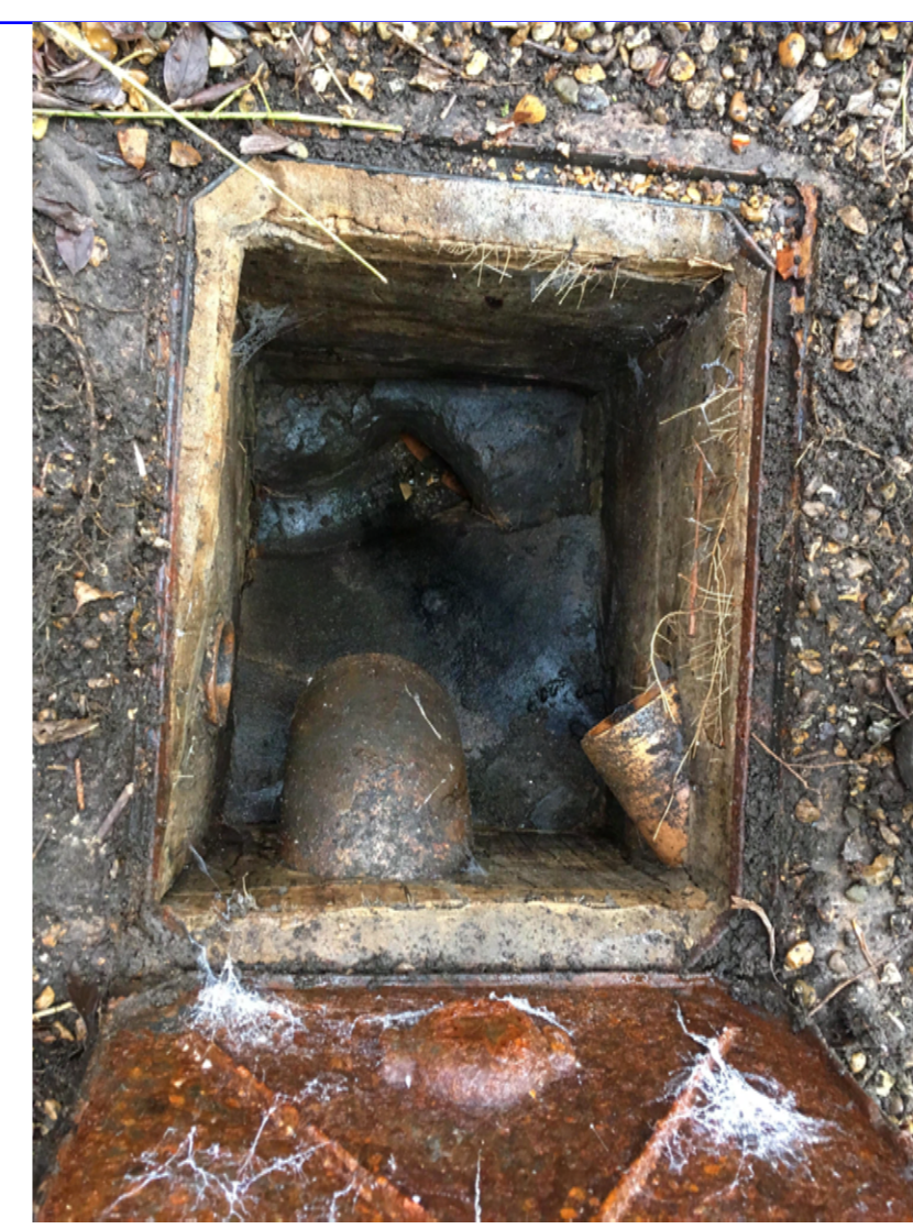
Existing Foul Connection
